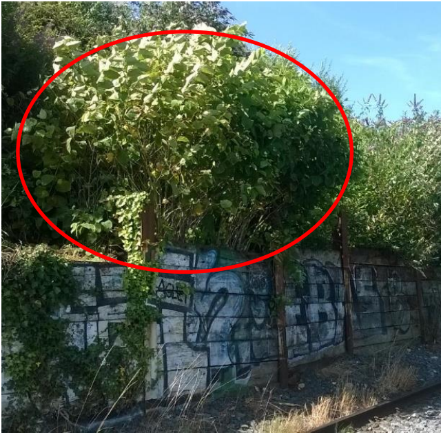
Photograph A1: Japanese knotweed recorded behind retaining wall south of the railway track during previous Irish Rail surveys
