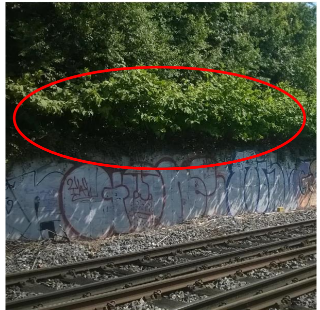
Photograph A2: Japanese knotweed recorded behind retaining wall at the boundary with Glasnevin cemetery during previous Irish Rail surveys
